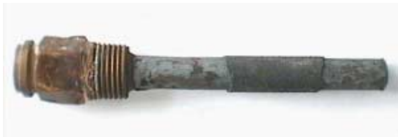
Fig. 5: Corroded casing for a thermocouple in a circuit treated with phosphate and sulfite, with deposits of \text{Cu}_2\text{S} .
